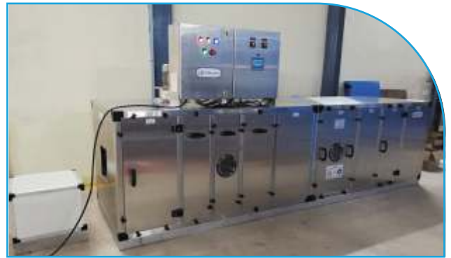
HVAC AND AIR HANDLING SYSTEMS
